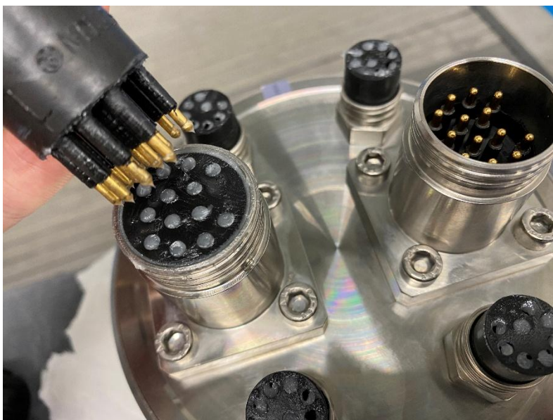
Above: Example of grease correctly applied to connectors
